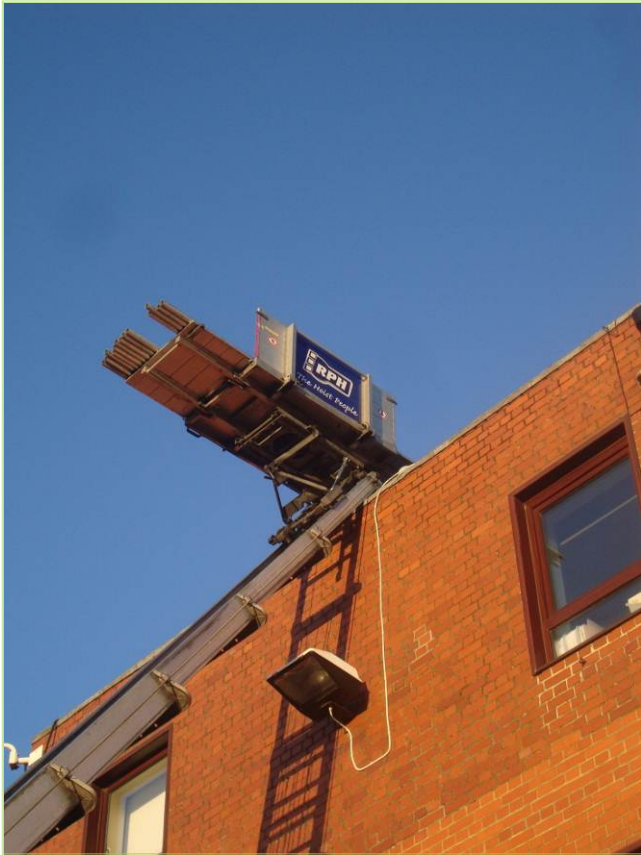
6m lengths of galvanized steel tube being taken to roof via vehicle mounted hoist
